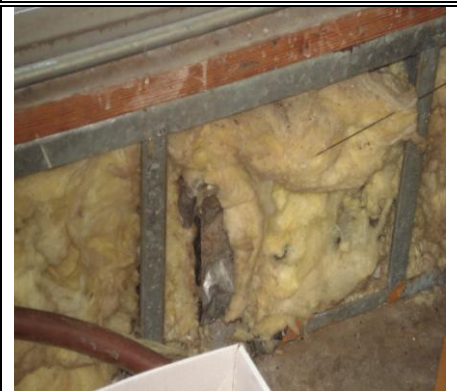
Insulation in the maintenance area needs to have a proper air barrier.
