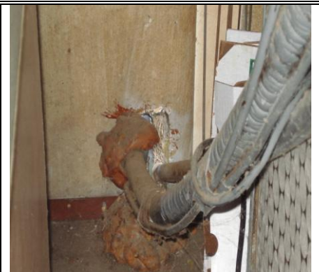
Holes for A/C lines have been foamed before but leakage still occurring.
