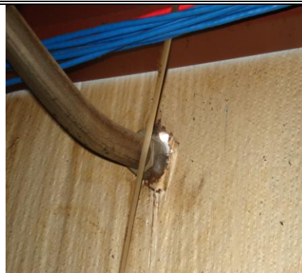
Hole for conduit is too large and needs spray foam.
