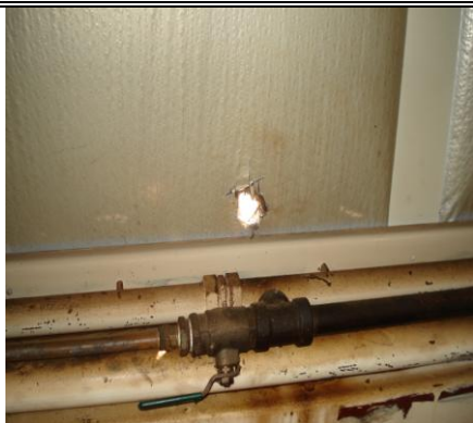
Hole penetrating outer envelope on the top deck needs sealing to prevent air exchanges.
