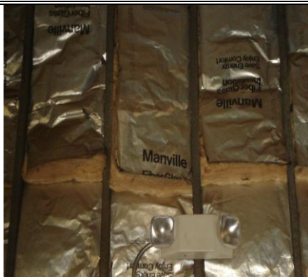
Insulation in maintenance shop needs proper placement and a better air barrier.
