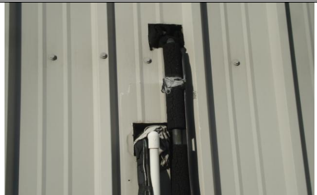
Large opening around refrigerant lines needs spray foam.
