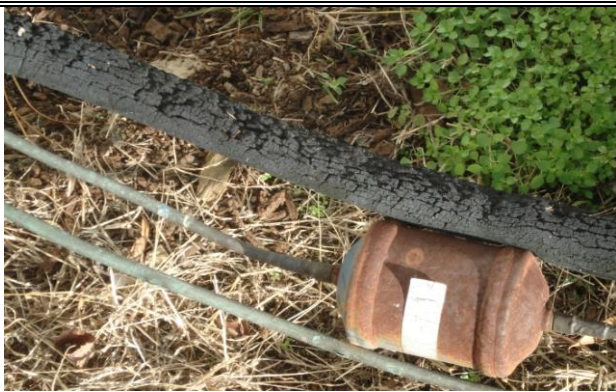
A/C refrigerant lines outside of ink department needs new insulation.
