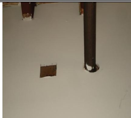
Several penetrations through wall that separates office and production areas needs sealing.
