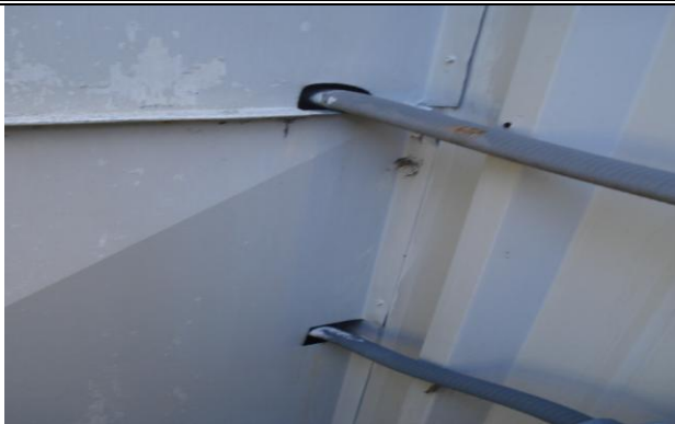
Holes through duct around conduit needs sealing with foam.
