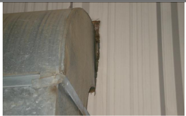
Large gap around supply duct for ink lab needs to be sealed with foam backing.
